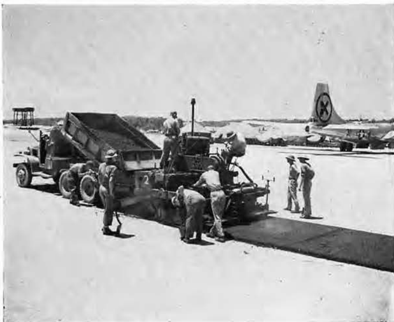
The asphalt plant is now in full operation and work commences on the runways. Many long hot days followed for the asphalt crews before the job was completed.
